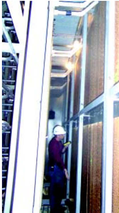
ABOVE: Evap inspector checks for gaps in the media and signs of deterioration.
