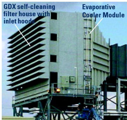
This Donaldson Evaporative Cooler enables this GE Frame 7FA Gas Turbine near Lubbock, Texas, USA, to yield maximum output even during the hot dry summer months.
