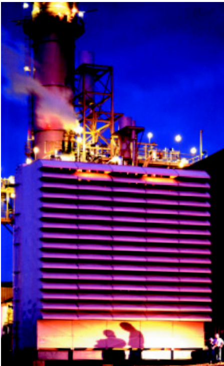
The Donaldson evaporative cooler, positioned behind the GDX self-cleaning air filter, reduces inlet air temperature for a Siemens Westinghouse 501FC Gas Turbine near St. Paul, Minnesota, USA.
