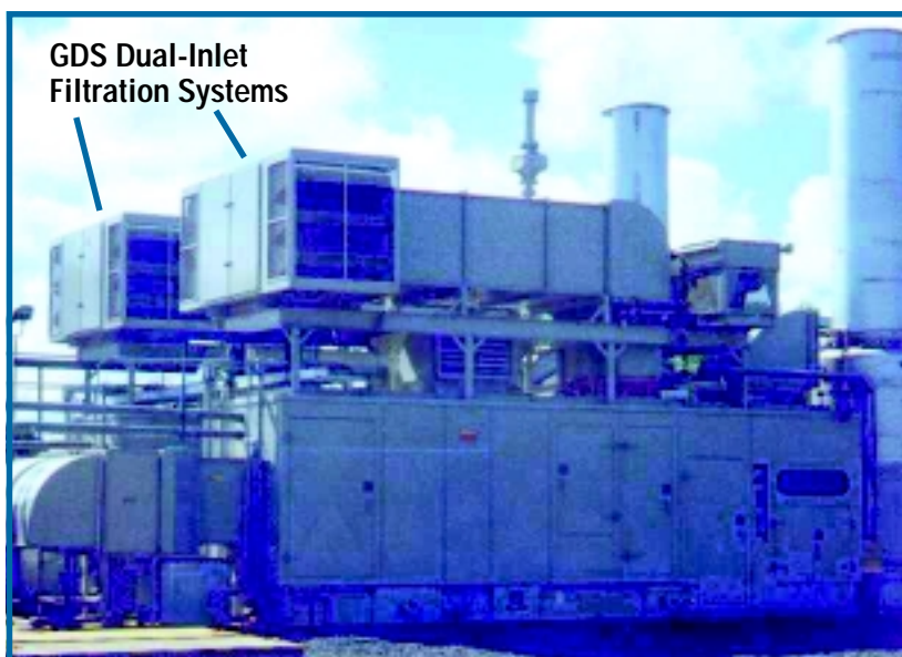
These Donaldson Dual-Inlet GDS Filter Systems protect turbines from the ravages of sand and dust near Tucson, Arizona USA. Note the insect screens over the inlet hoods. Donaldson GDS systems keep combustion air clean for hundreds of turbines all over the world.
